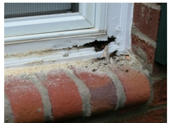
ROTTING BRICKMOULD (WINDOW WAS MOUNTED INTO OPENING IN PHOTO ABOVE)
