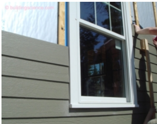
Siding butted directly to brick-moulding
